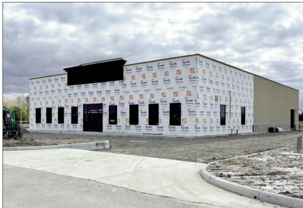
Caliber Collision has an 11,000-square-foot building under construction on a Meijer out lot off Conant Street.
